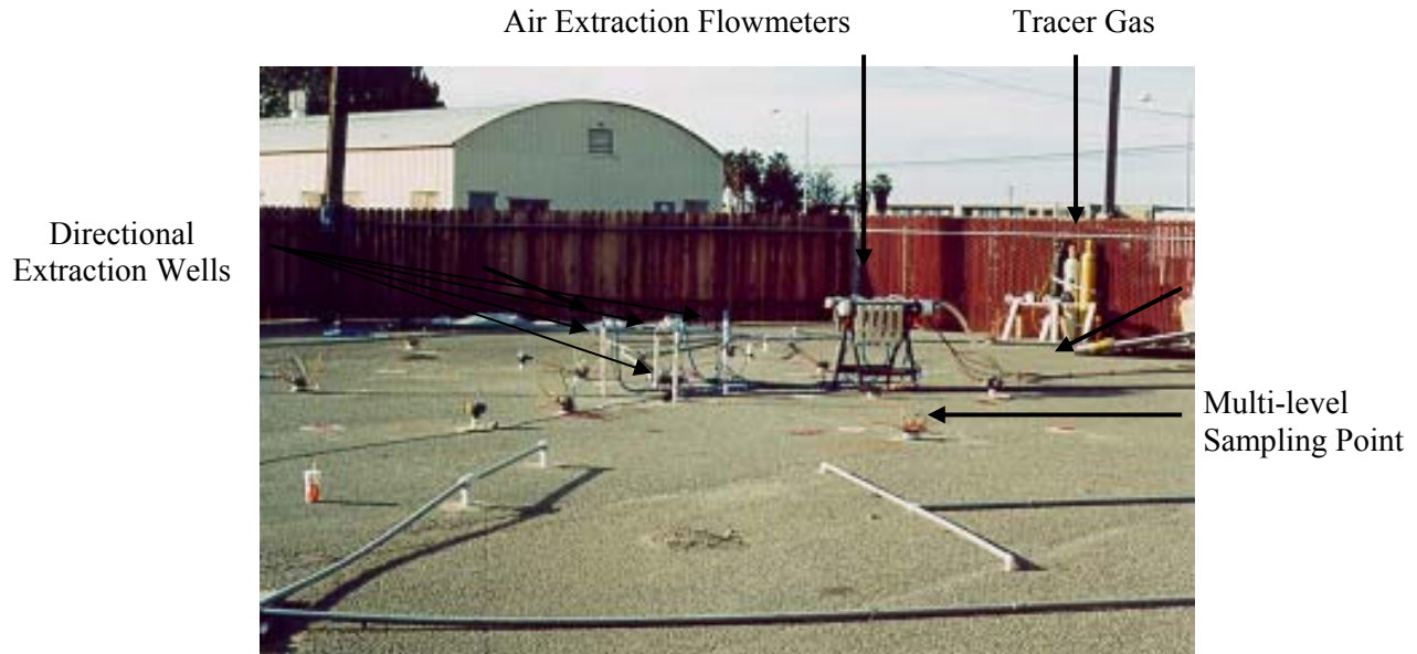
Figure 6. The Single-Well Pilot Test Air Sparging Setup at Site 1
