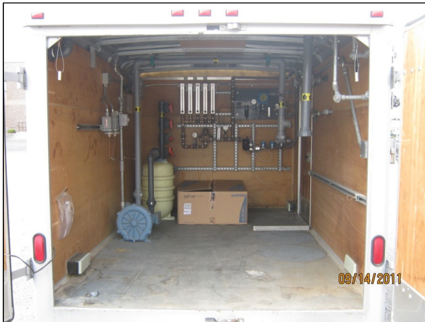
Figure 5-20. Inside of Trailer # 2, which houses the propane feed and distribution as well as SVE equipment.
