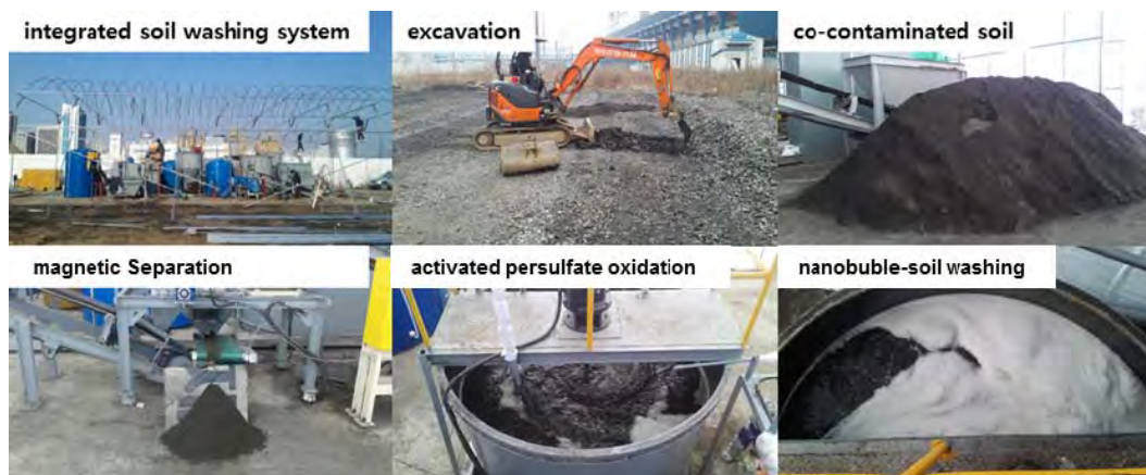
Fig. 1. The integrated soil remediation system
